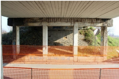
Figure 4: Details of deterioration of the bridge.
