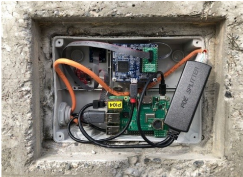
Figure 9: The prototype of SAB1 installed on the renovated bridge. SAB1 is equipped with a triaxial accelerometer and a biaxial inclinometer.
