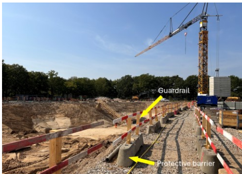
Figure 5: Installation of protective barrier to separate pedestrian worker walkway from vehicle traffic.
