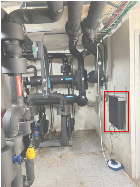
Figure 4: Edge computing solution 1 installed in the hotel substation in Montserrat
