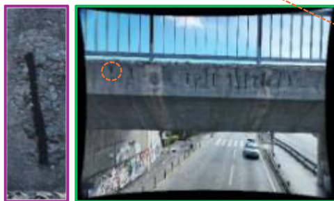
Figure 10: the "as-damaged" BrIM model visualizing mapped defects (light blue) alongside the associated property window displaying quantified dimensional attributes (e.g., area, length) and links to the source reference image and generated orthophoto.
